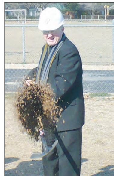
Bishop Kevin Vann breaks ground, turning a shovel of soil to begin construction on St. Andrew School's 5,983-square-foot, $800,000 kindergarten building.
