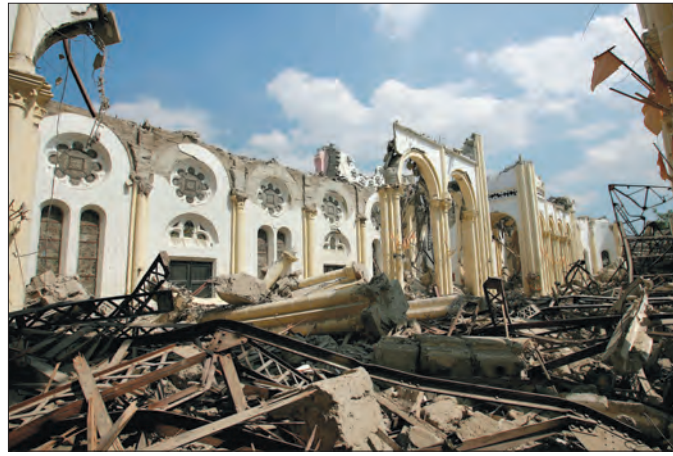
An interior view of the destroyed Cathedral of Our Lady of the Assumption is seen in Port-au-Prince, Haiti, in early February. (CNS photo/Bob Roller)
