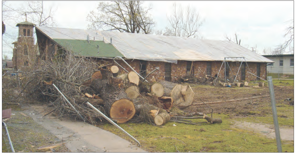
Plastic covers the damaged St. Agnes parish hall roof. St. Agnes Church, though structurally sound, was hit hard by the Mena tornado April 9. The worst damage came from a large oak tree that fell between the church and rectory, knocking part of the eaves away, exposing a gap between the roof and ceiling of the church. The storm also blew off several roof tiles, damaged a stained glass window, bell tower louvers and bent a metal cross on the roof.
