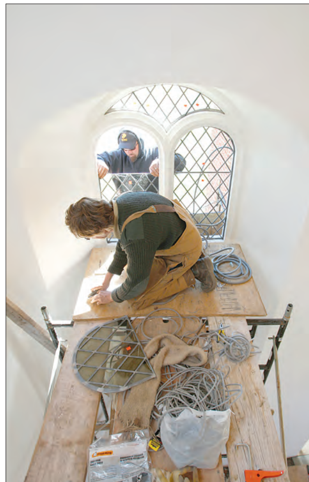
Peter Rivers, front, and Berkley Taylor, prepare to install a window during the reconstruction of the 1667 brick chapel in the Chesapeake Bay region. (CNS photo/Bob Roller)
