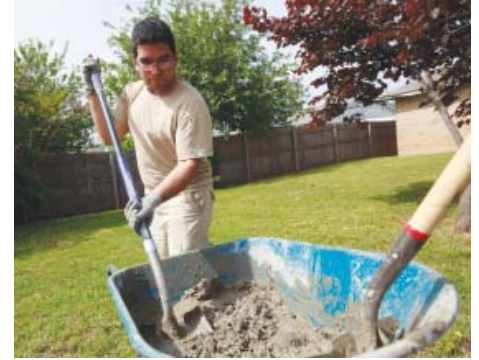
Matthew Moreno mixes concrete at one of the FIAT team’s work sites on May 13.
