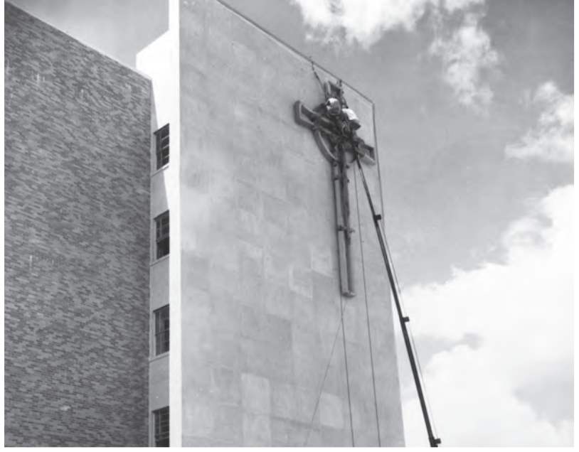
Workers install a cross outside of St. Joseph Hospital in 1958. (Fort Worth Star-Telegram Collection, UTA Libraries)
