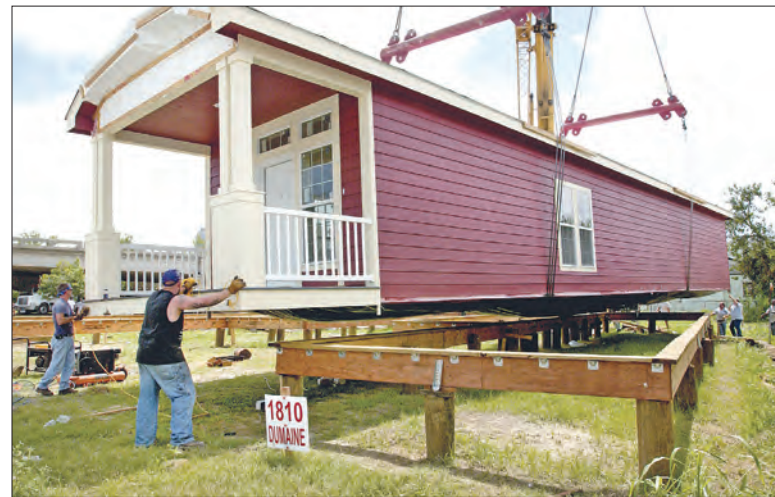
Workers from Palm Harbor Homes in Austin move a modular house into position in a housing development in New Orleans Aug. 17. The lot is owned by St. Peter Claver/Ujamaa Community Development Corporation. It is an example of what the Catholic-run Providence Community Housing initiative wants to do with 196 blighted properties it has acquired from the city of New Orleans. Providence hopes to build, rehab, or operate 7,000 housing units in the next five years. (CNS photo/Peter Finney Jr., CLARION HERALD)
