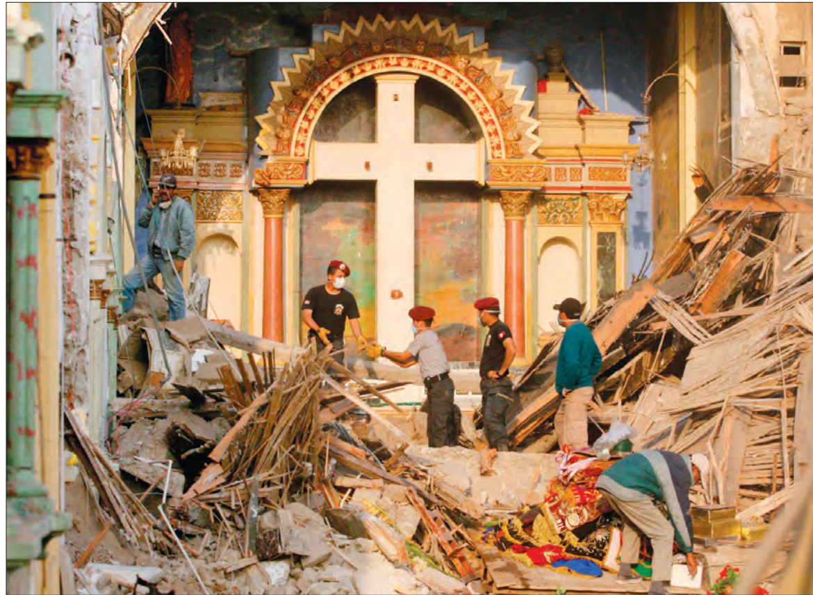
PERU EARTHQUAKE RECOVERY — Peruvian workers recover items from an earthquake-destroyed Catholic church in Pisco, Peru, Aug. 19. More than 500 people are known to have been killed and 1,500 injured in a magnitude 8 earthquake that struck about 125 miles south of Lima Aug. 15. (CNS photo/Mariana Bazo, Reuters)
