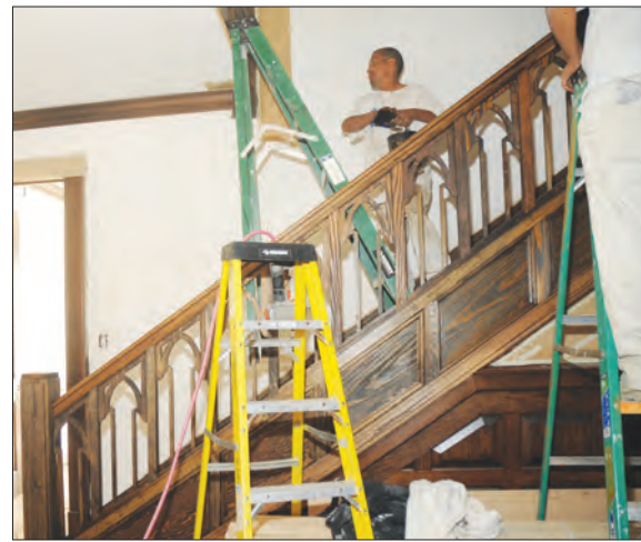
Throughout the renovation process, several aspects of the building were uncovered, such as this part of the rectory's original staircase.
