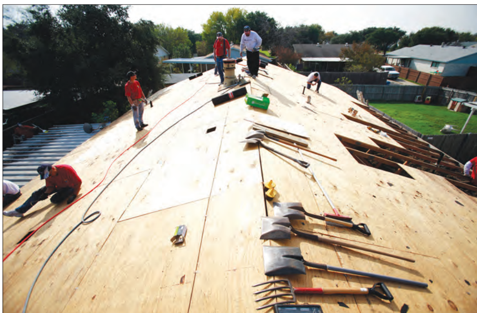
Knights of Columbus Council 8493 from Holy Cross Parish helped to put a new roof on Virginia Fraser's home. Fraser, a widow who is legally blind, she cares for her 12-year-old granddaughter. Fraser faced losing her home, but Richard Anderson, a local lawyer and Knight helped her save it. The Knights' efforts allowed her to get home insurance.
