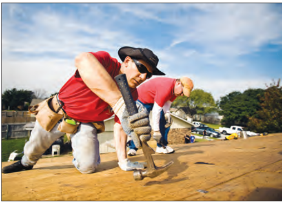
James De Piazza, a local judge, takes out old nails from the roof.
