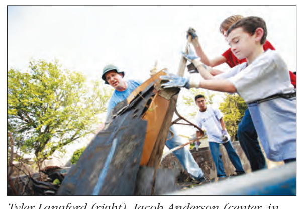
Tyler Langford (right), Jacob Anderson (center, in red) and their youth leader Calvin Wolf (left) helped dump old shingles and roofing material.
