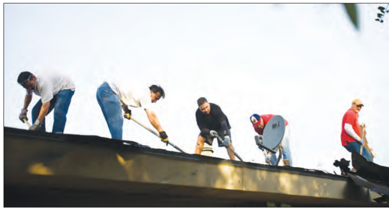
Several Knights and parishioners from Holy Cross parish helped to put a new roof on a fellow parishioner's home.
