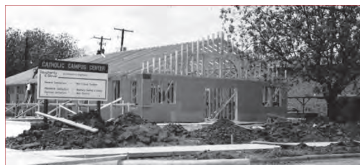
Construction on the Midwestern State University Catholic Campus Center begins in early 1986. Photo courtesy of MSU CCC
